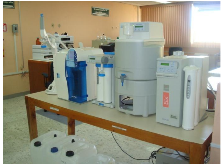
Water Purification System
