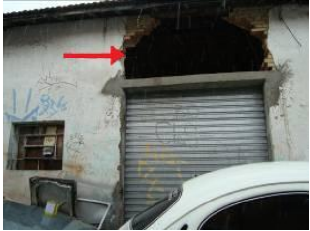
Fig 2. Front of the automotive body repair workshop. In detail (red arrow), the broken piece on the wall between the door and ceiling, being the only way of ventilation.
