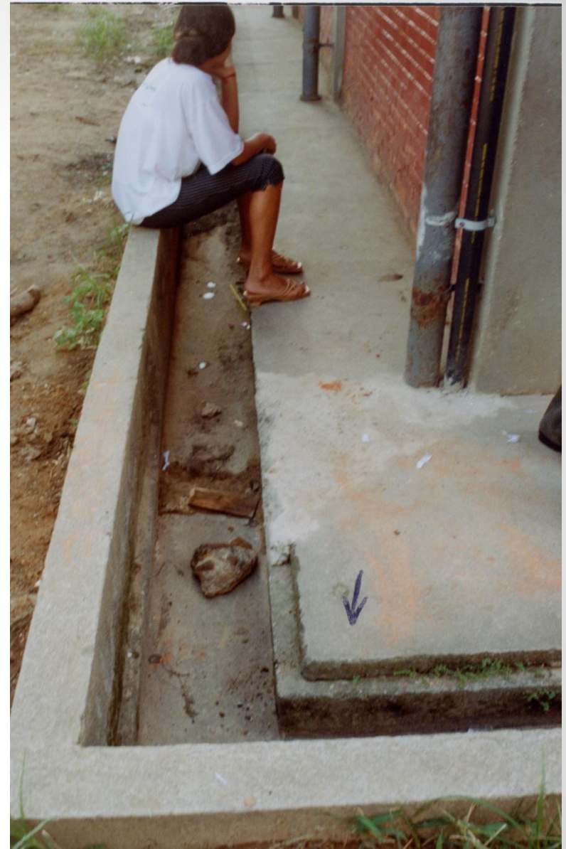
Figura 4 – Absence of grating in the gutter of pluvial water.
